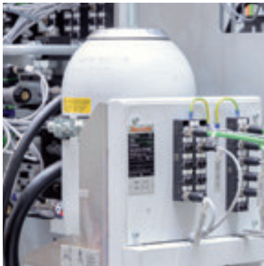
Pressure accumulator hydraulic unit
